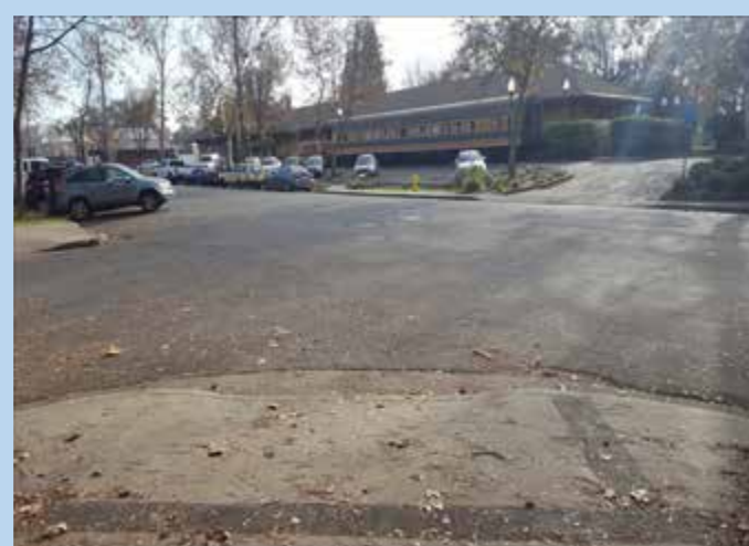
Current existing ramps are not ADA compliant and lead directly to the middle of intersection.
