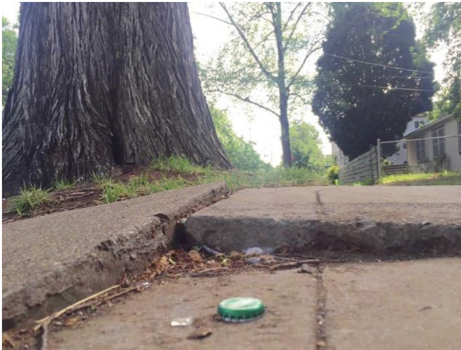
Figure 21: Example of sidewalk uplift. (Photo by S. Roe)
